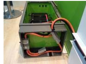
Housing for Cabling
